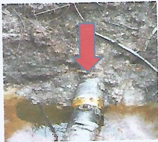
Pic1: Showing one (1no.) 2" nipple illegally installed on the pipeline
